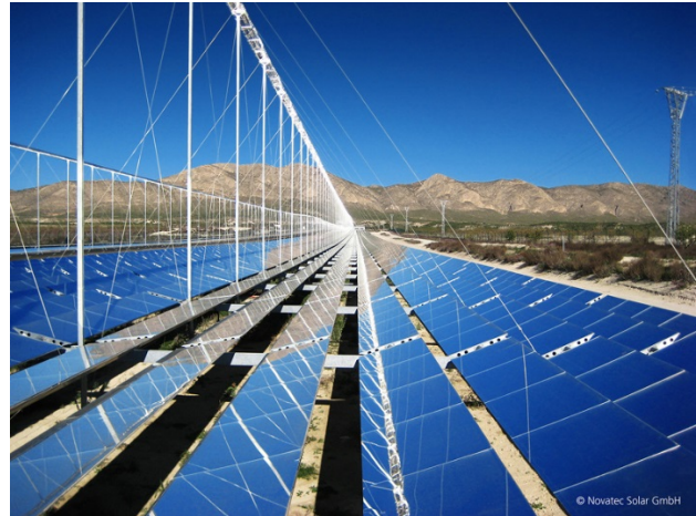
Figure 1. Field of mirrors in a Fresnel plant (source: Novatec Solar GmbH). What are optimal mirror sizes and positions? How high does the pipe have to be?
