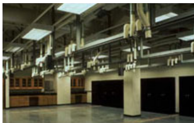
Figure 1. Building Attributes: Labs designed with overhead connects and disconnects allow for flexibility and fast hook up of equipment.
