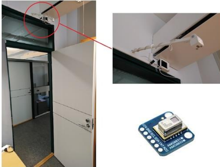
Fig. 1. The sensor and Raspberry Pi mounted above a doorway. Sensor mounting height is typ. 2.4 m and the room height is 3.24 m. Door is a standard size of 0.8 m x 2.0 m. AMG8833 sensor board is shown on the bottom right.
