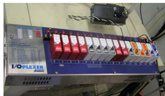
Figure 4. Ioplexer control modules 1
