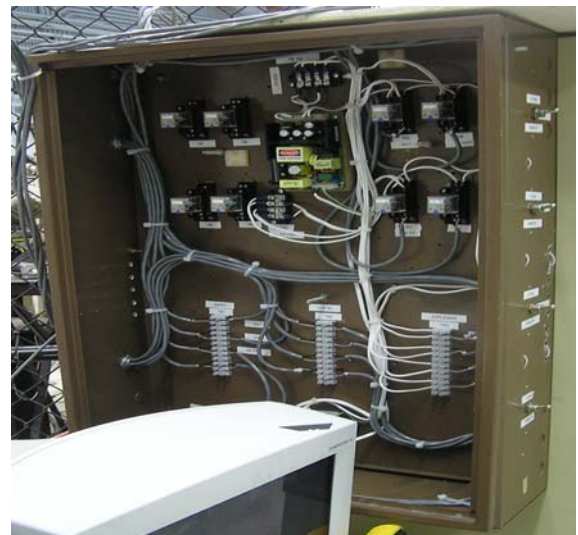
Figure 6. Relay control box 1
