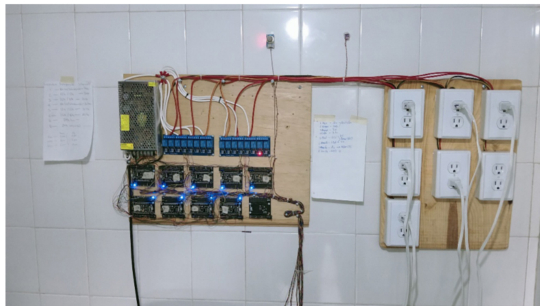
Fig. 5. Incubators centralized control panel
