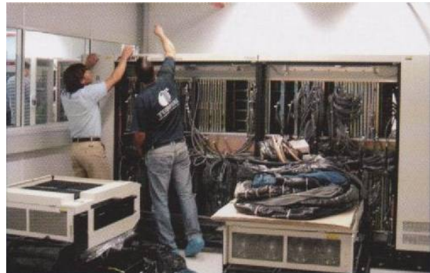
Figure 2. T5365 installation and set up at Qimonda.
