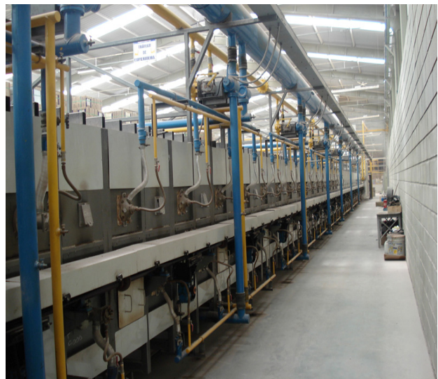
Figure 1. Photo of the roller hearth kiln installed at AngelGres.
