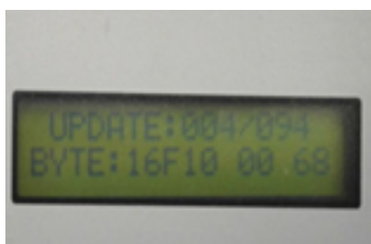
Figure 16. Display of RTU
