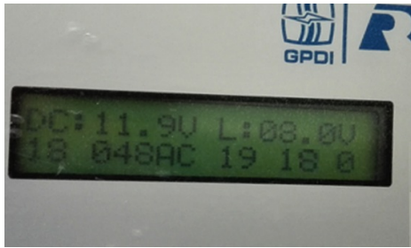
Figure 13. Display of RTU
