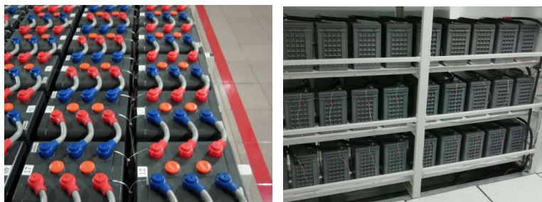
Fig. 1. The different ways of energy storage battery grouping
